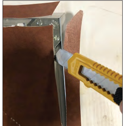
Make sure to trim off any excess banner material off the outer edge of the tacky area by inserting a box cutter knife into the channel and cutting off. This is important so that excess banner does not interfere with the CAP top rail installation.
